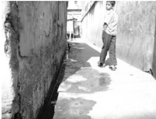
Fig. 4: Open drain with low capacity
