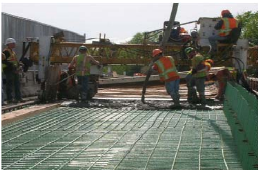
Figure 2. Internally cured concrete being cast at Bartell Road in New York (Wolfe, 2010)
