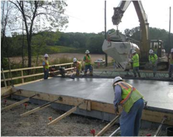
Figure 3. Internally cured concrete bridge deck being cast near Bloomington, IN (Di Bella, Schlitter, & Weiss, 2010)
