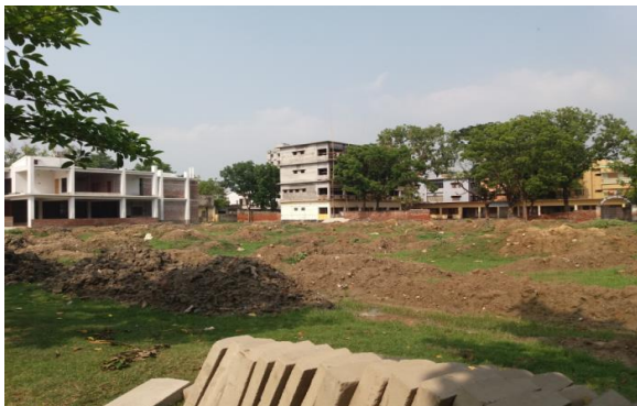
Fig. 8: Land fill-up with soil in Upashohor Secor-2 open space in RCC area.
