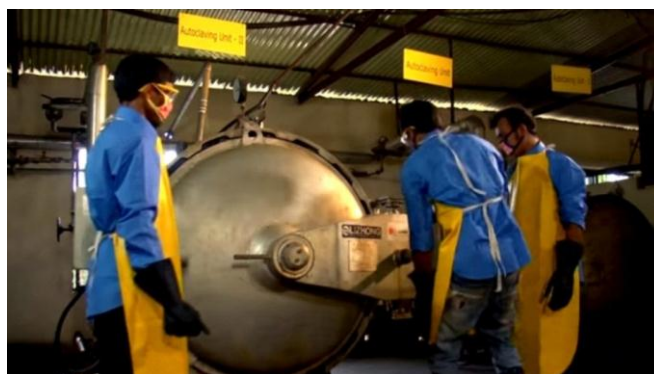
Figure 06: Autoclaving system Source: PRISM Bangladesh, 2017
