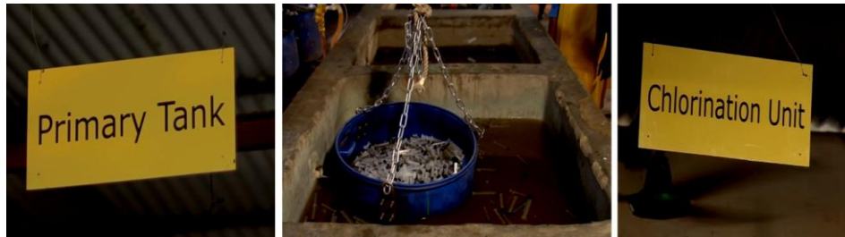
Figure 09: Chemical disinfection system
