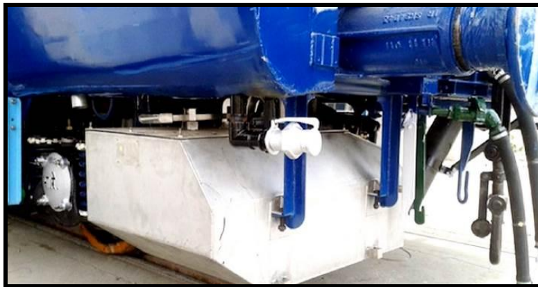
Figure 2 Bio Toilet System in Train
